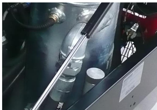
Figure 10.1-1 Checking the oil level in the compressor
